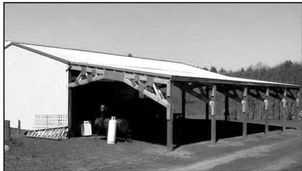
Following the collapse of the sale tent in a last winter's ice storm, volunteers helped Arlen Aleckson add a sturdier extension to the haybarn.
