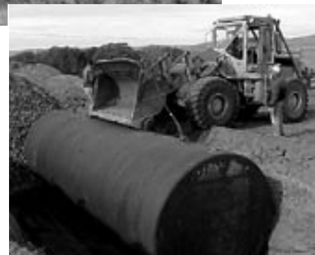
Above: Loading tank on Schilling Road prior to move to Struck Road.
